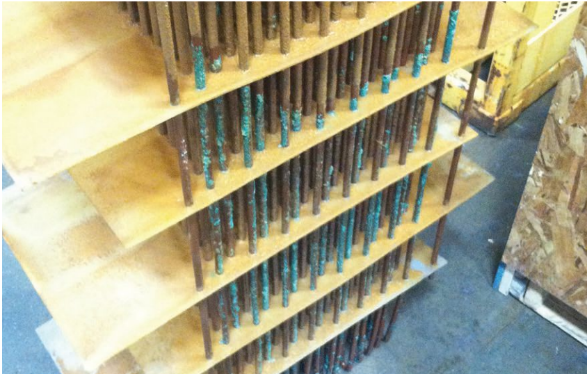
The green seen on this evaporator coil is calcium buildup, which prevents the heat transfer from water into the refrigerant.
